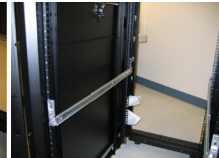
Figure 5C: IBM mounting rails in rack.
