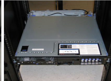
Figure 6C: IBM server in rack.
