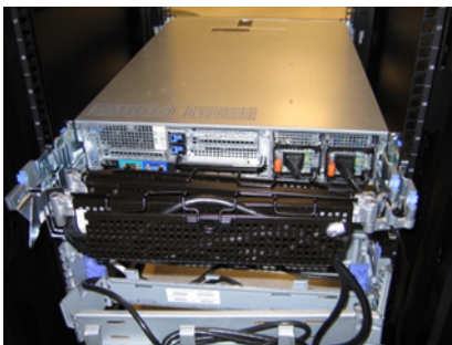
Figure 7A: Dell cable management system and power cords.
