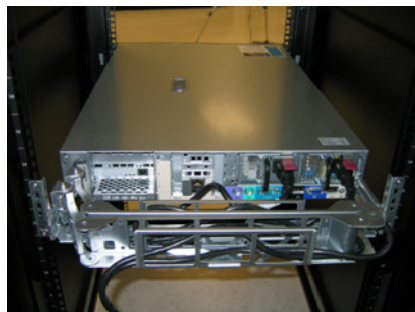
Figure 7B: HP cable management system and power cords.
