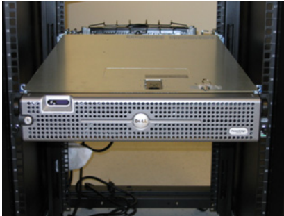
Figure 6A: Dell server in rack.
