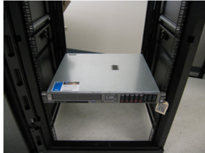
Figure 6B: HP server in rack.
