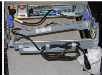
Figure 7C: IBM cable management system and power cords.
